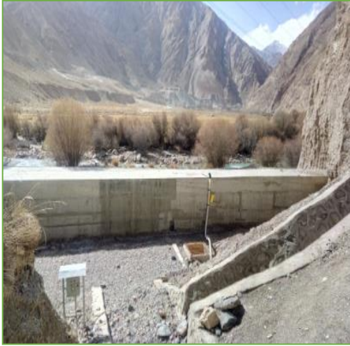
50m 3 渗滤液收集池及下游截渗墙
